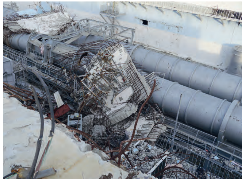
Fig. 2.5.3. Debris from the upper levels of unit 4 at the Fukushima Daiichi power plant in December 2012, 21 months after the nuclear accident.
