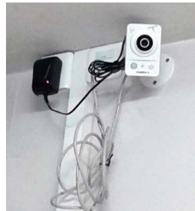
Fig. 14. Video monitoring in liquid nitrogen facilities.
