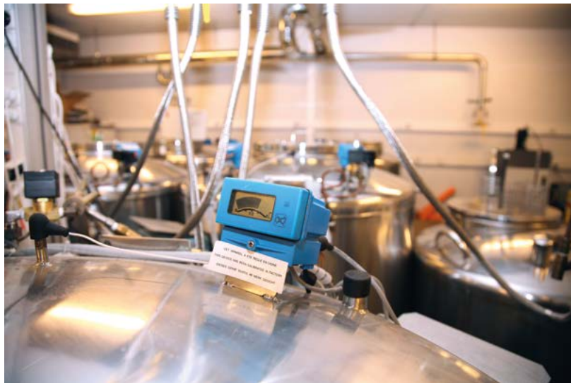
Fig. 13. A tank fitted with a monitoring device, which shows the level of liquid nitrogen inside the tank.
