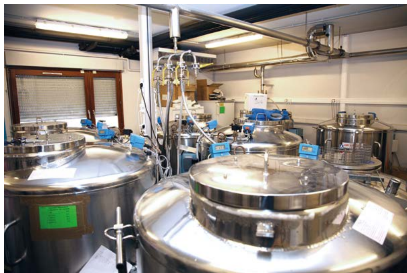
Fig. 5. Liquid nitrogen facility with \text{LN}_2 tanks.
