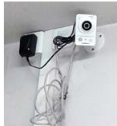
Fig. 14. Video monitoring in liquid nitrogen facilities.
