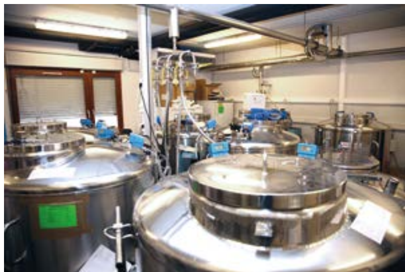
Fig. 5. Liquid nitrogen facility with \text{LN}_2 tanks.
